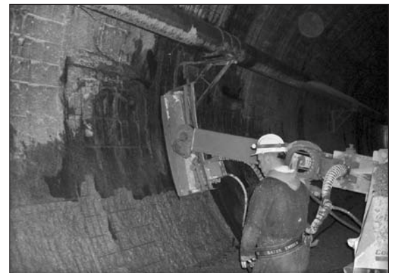
Conjet supplied specially modified banana-shaped feedbeams, which carried the jetting nozzle, to match the curvature of the tunnel wall.
