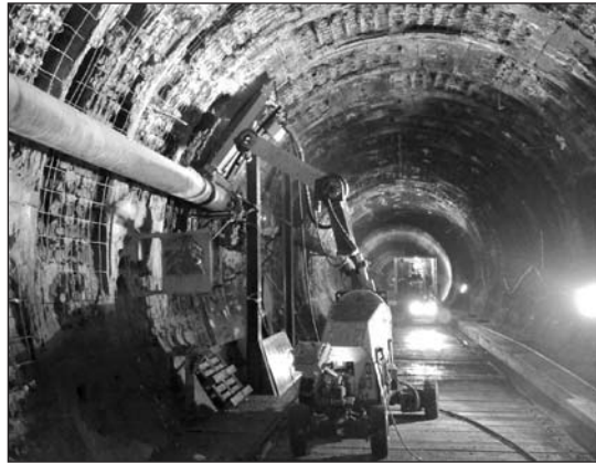
The total area of removal of the fire damaged concrete was about 9,500m 2 over an approximate 600m length of tunnel, including about 350m 2 directly above where the fire damage was most severe.
