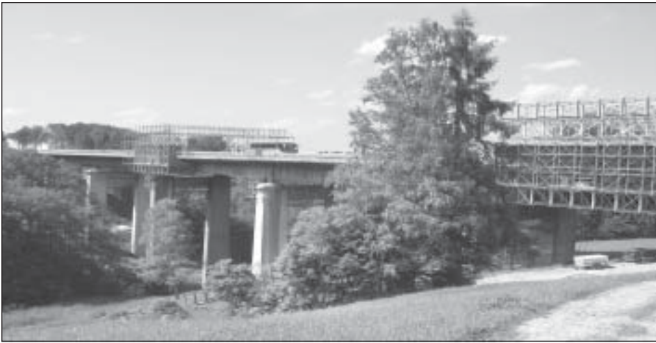
The 286 m long Loithal Bridge on Germany's A8 autobahn was experiencing corrosion problems with rebar along the parapet caused by salt laid over the winter months to combat the heavy snowfall.
