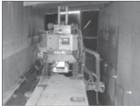
Two hydrodemolition robots from Aquajet enclosed within a gantry above the parapet on both sides of the bridge are removing more than 140m 3 of badly corroded concrete.
