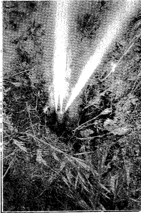
FIG 18 WATER JET DRILL BIT EXITING ON GROUND SURFACE FROM TUNNEL 60 FEET BELOW
