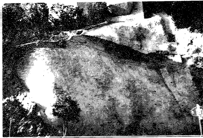
FIG 7 COMPLETED CLIFF STABILIZATION USING WATER JET DRILLING TECHNIQUES SEVERAL YEARS AFTER COMPLETION
