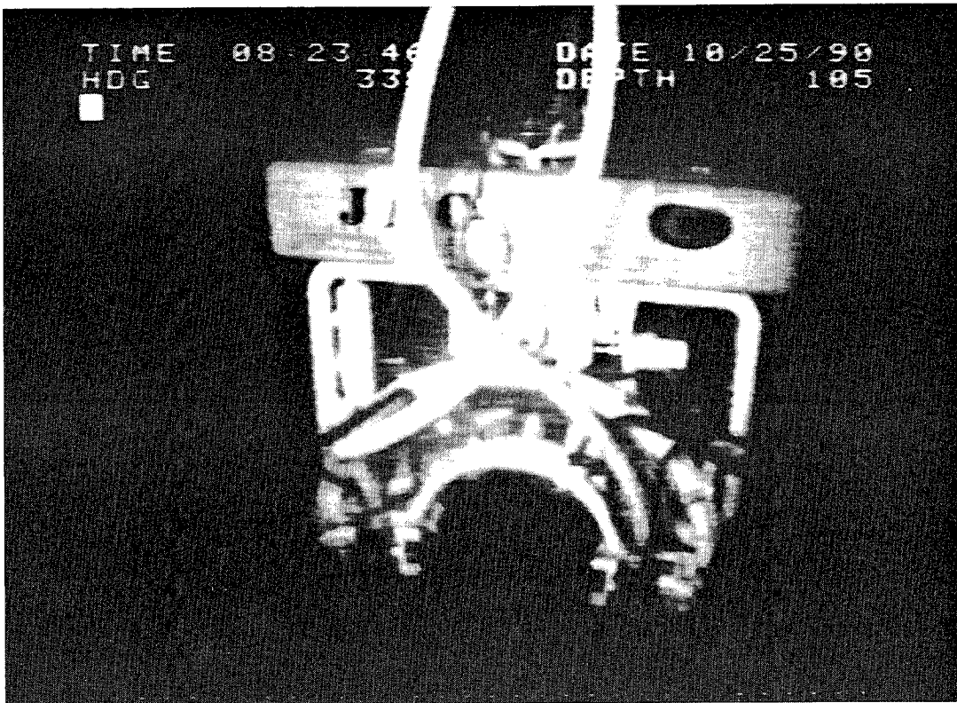
Fig 5 Comex Jet Abrasive Clamp operating 105m sub-sea off Norway cutting a pipeline with two DIAJET nozzles
