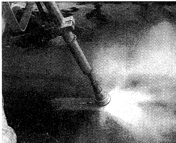
Figure 18. Weld inspection and testing is possible following paint and coating removal using 36,000 psi water, which produces a “white metal” surface.
